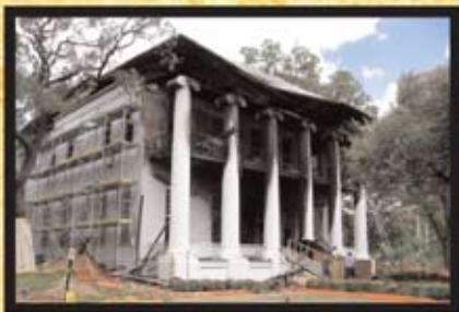
After the fire on June 8, 2008.
